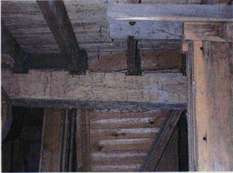
Photograph 7: Joists lifted from their bearing positions due to jacking of the floor system.
