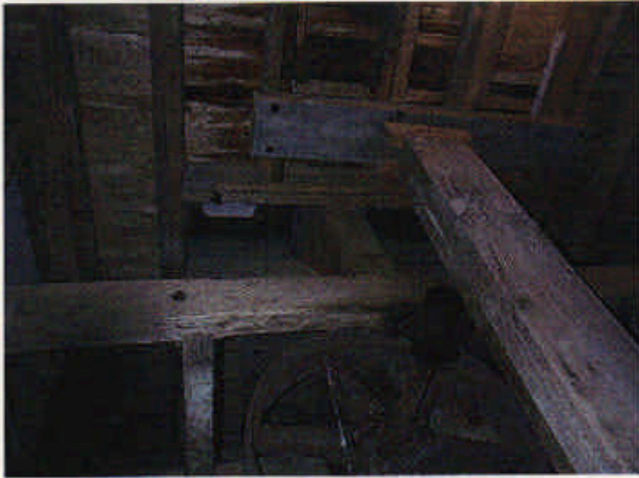
Photograph 5: Additional column and framing in the hopper area.
