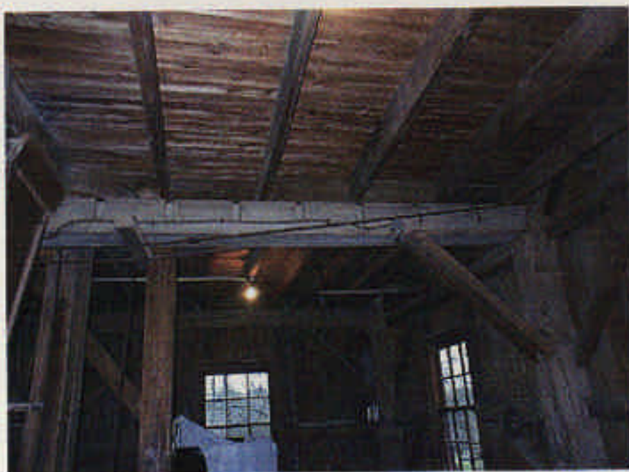
Photograph 3: Mezzanine floor framing. Note the notching of the beam at 16" o.c. where the joists are placed at 2'-0" o.c.
