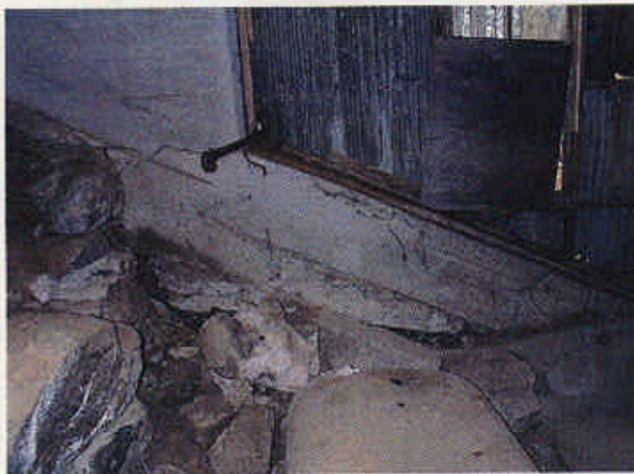
Photograph 10: Crack in existing concrete foundations. Note the loss of bearing under the footing indicating large footing movements.
