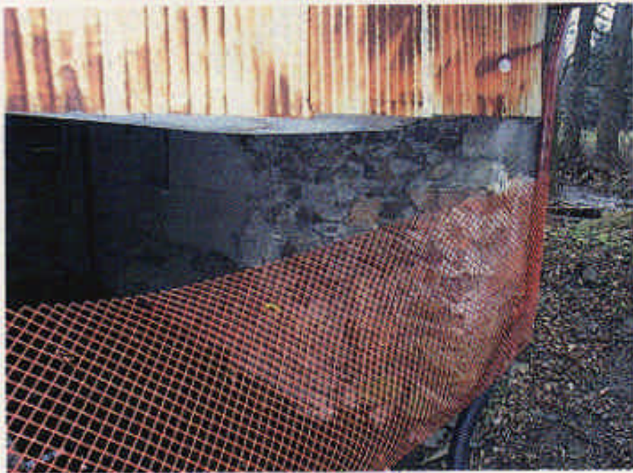
Photograph 9: Partial collapse of the rubble stone foundation in the spillway.
