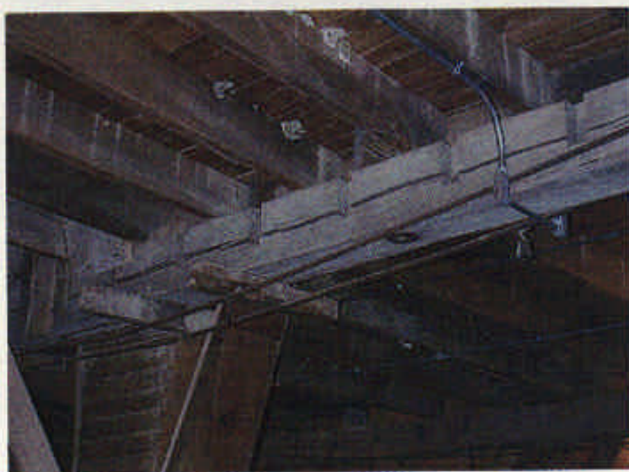
Photograph 4: Large crack in existing beam. Note the steel reinforcing rod in the existing beam.
